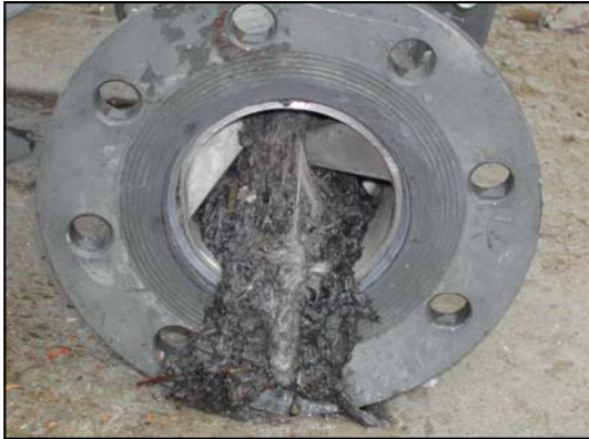
Typical clogging of competitors static mixer in less than 4 hours
